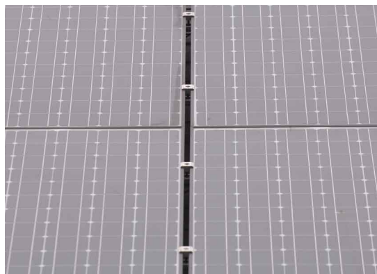
Roof-top electricity generator – the Pilcher's photovoltaic panels
