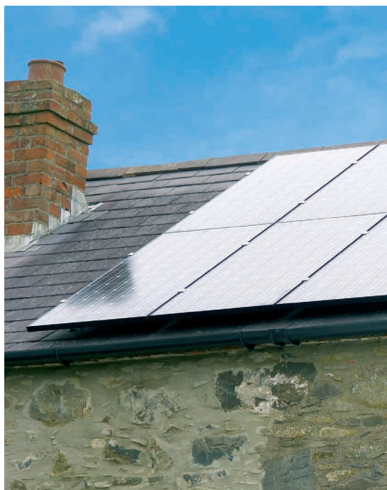
Photovoltaic panels are a perfect match for Pilcher's slate roof.
