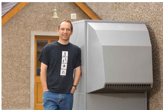
Where there's air, there's heat. David Simpson and his air source heat pump.
